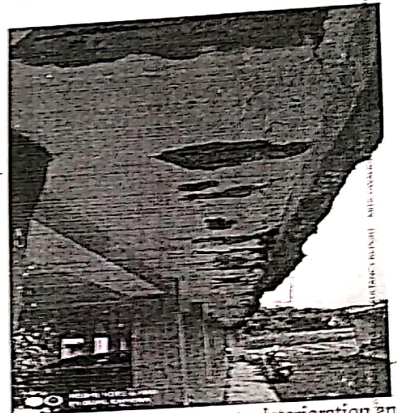
Photo 26: Excessive concrete deterioration and reinforcement exposure in the ceiling of car parki
