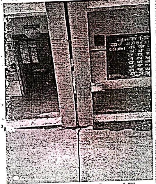
Photo 6: Open joint at Ground Floor
