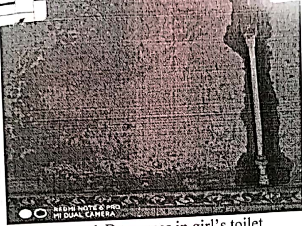
Photo 1: Dampness in girl's toilet
