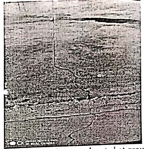
Photo 8: Cracking on the stage located at ground floor
