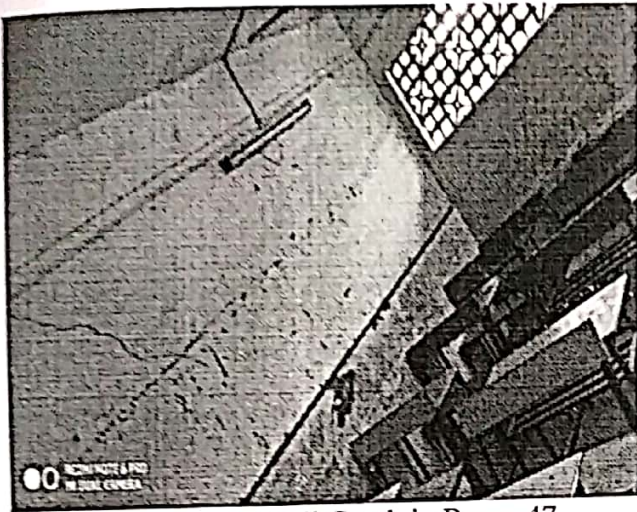
Photo 7: Big Wall Crack in Room 47
