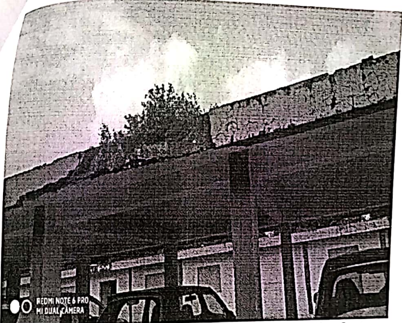
Photo 27: Spalling of concrete in the roof slab of car parking
